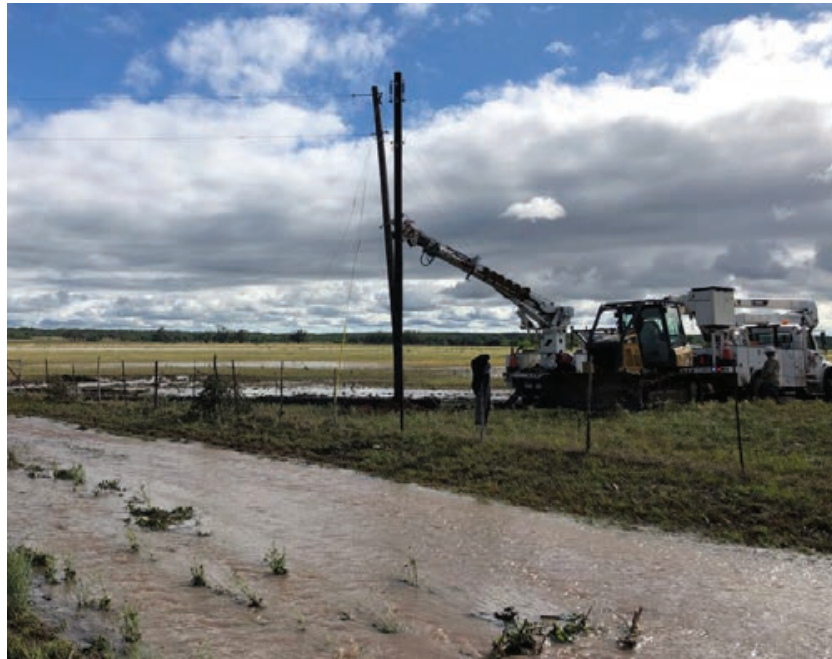
MEDINA EC CREWS WORKING TO RESTORE POWER AFTER SPRING STORMS AND TORNADO HIT MEDINA COUNTY IN APRIL 2021.
