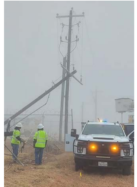
DILLEY CREW MEMBERS RESPONDING TO AN OUTAGE CAUSED BY A CAR ACCIDENT IN JANUARY.
