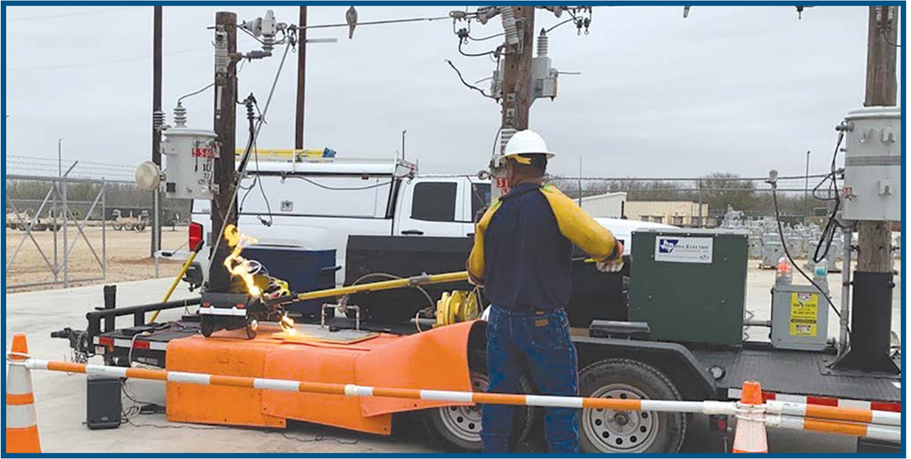
TONY BANDA, AREA LINE FOREMAN IN THE DILLEY OFFICE, DISPLAYS AN ELECTRICAL ARC DURING A SAFETY DEMONSTRATION WITH THE LIVE LINE TRAILER.
